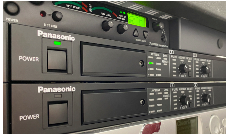
The WX-SR202 digital wireless receivers are rack mounted in locked cabinets outside of the classroom.
